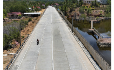
Upgrading works along a major road and a farm-to-market road (FMR) to facilitate a safer and more convenient travel in the municipality of Nueva Valencia, Guimaras.
