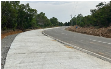
The widening activities are being carried out along specific locations of Guimaras Circumferential Road and Guimaras Central Road, as well as the improvement of local roads connecting local communities.
